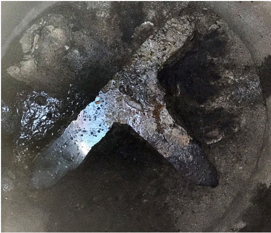
Grease-blocked sewer pipes
