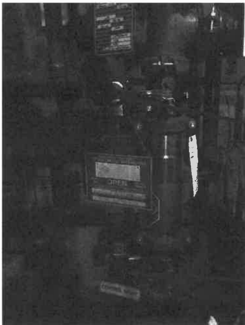
Sprinkler System Riser
