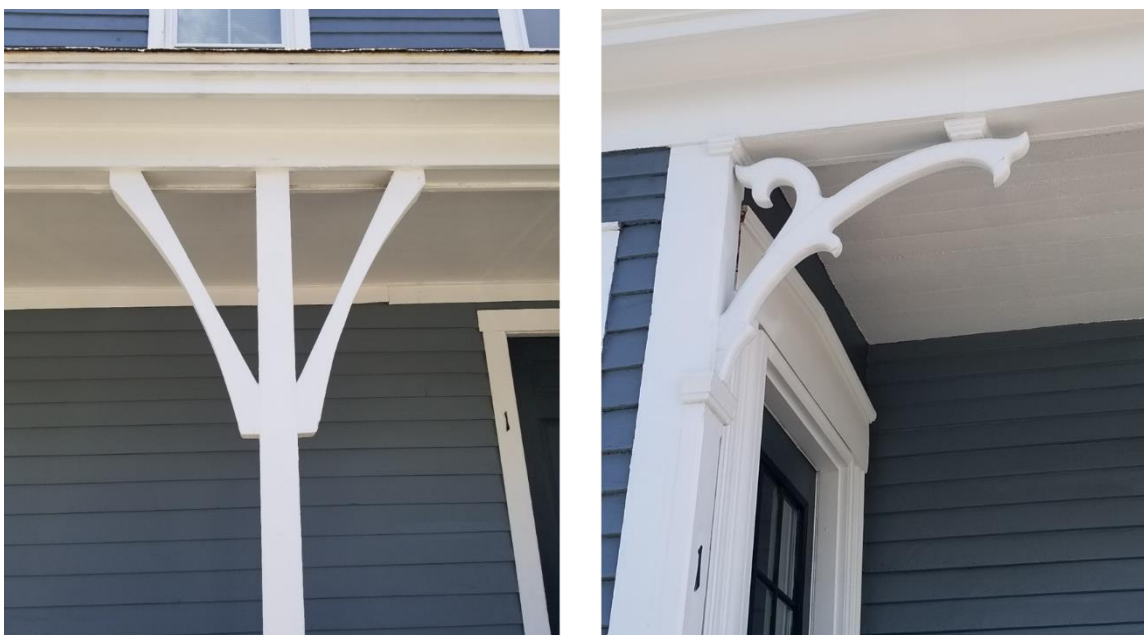
Figure 3. Photos submitted by the Applicant that show the wood trim features that will be preserved with encapsulating paint. These trim features are present on the porches on the east side of the 23 Mechanic Street building (left image) and the 17-19 Mechanic Street building (right image).
