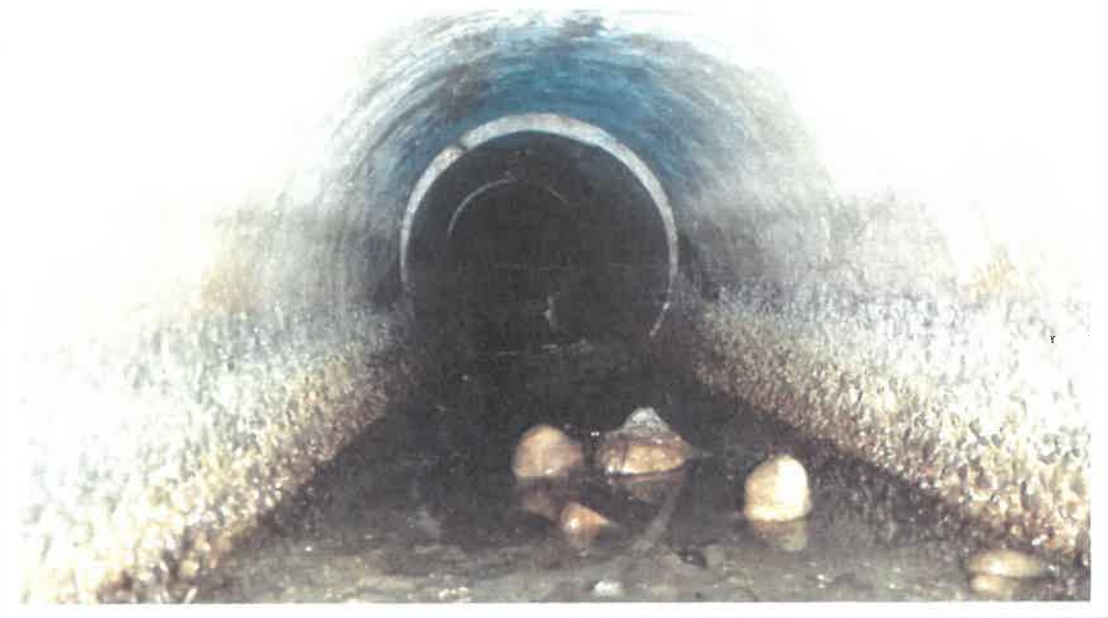
15" RCP Outlet – Joint Separation
