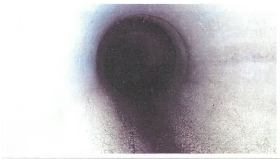
15" RCP Outlet – Joint Separation
