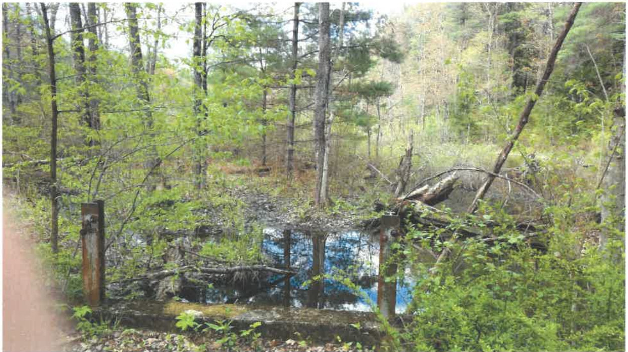
Wetland D above box culvert on main access road, looking north (no impacts)
