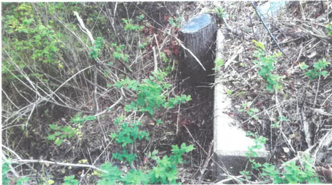
15" RCP Outlet and Headwall – Southern Bank of The Branch
