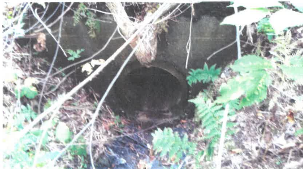
18" RCP Outlet and Headwall– Southern Bank of The Branch
