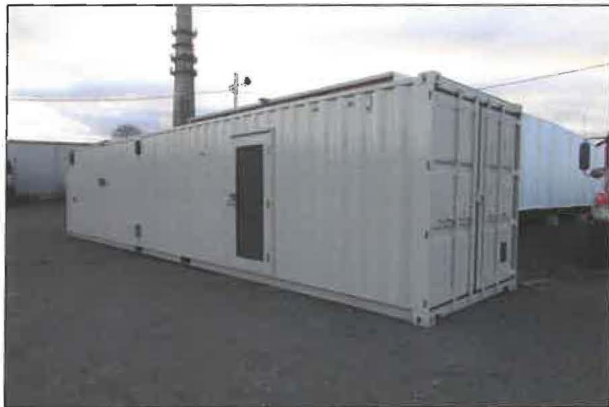
Figure 1: Decompression skid used in CNG facilities.
